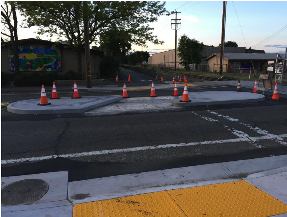
IN-PROGRESS INSTALLATION OF NEW PEDESTRIAN SAFETY ISLAND AT GOBBI STREET RAIL TRAIL CROSSING
