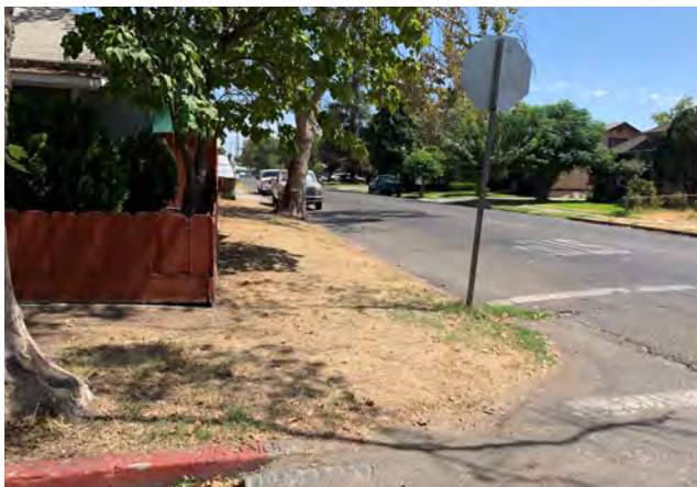
Top Left: Missing curb ramps on the southeast corner of High Street/Lane Street intersection.
