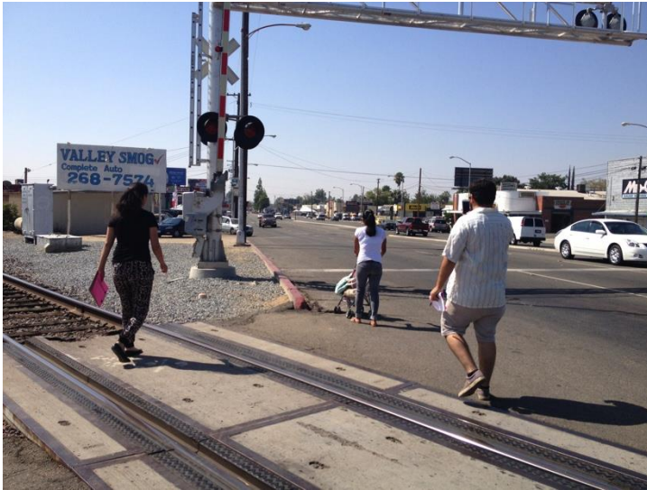
SIDEWALK ABRUPTLY ENDS ON EITHER SIDE OF RAILROAD CROSSING ALONG BLACKSTONE AVENUE FORCING PEDESTRIANS
