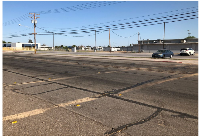
Marked but faded uncontrolled crosswalk on Main Street in front of the Calipatria High School and Fremont Primary School access lot.
