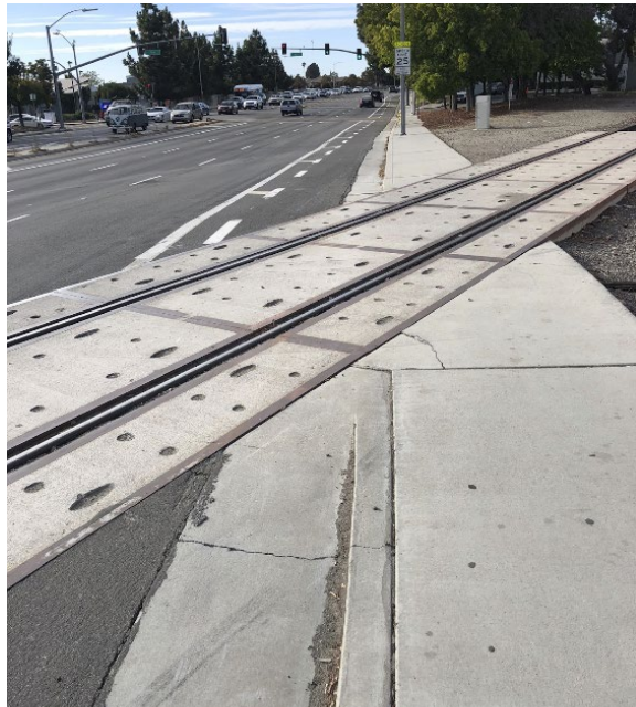
The severe angle of the railroad tracks on the east side of Oakland Road and lack of markings or signage create challenging conditions for bicyclists.
