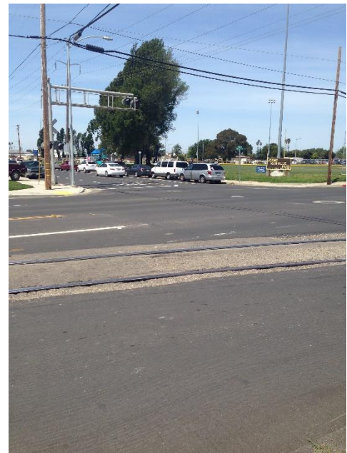
Uneven pavement due to train tracks.
