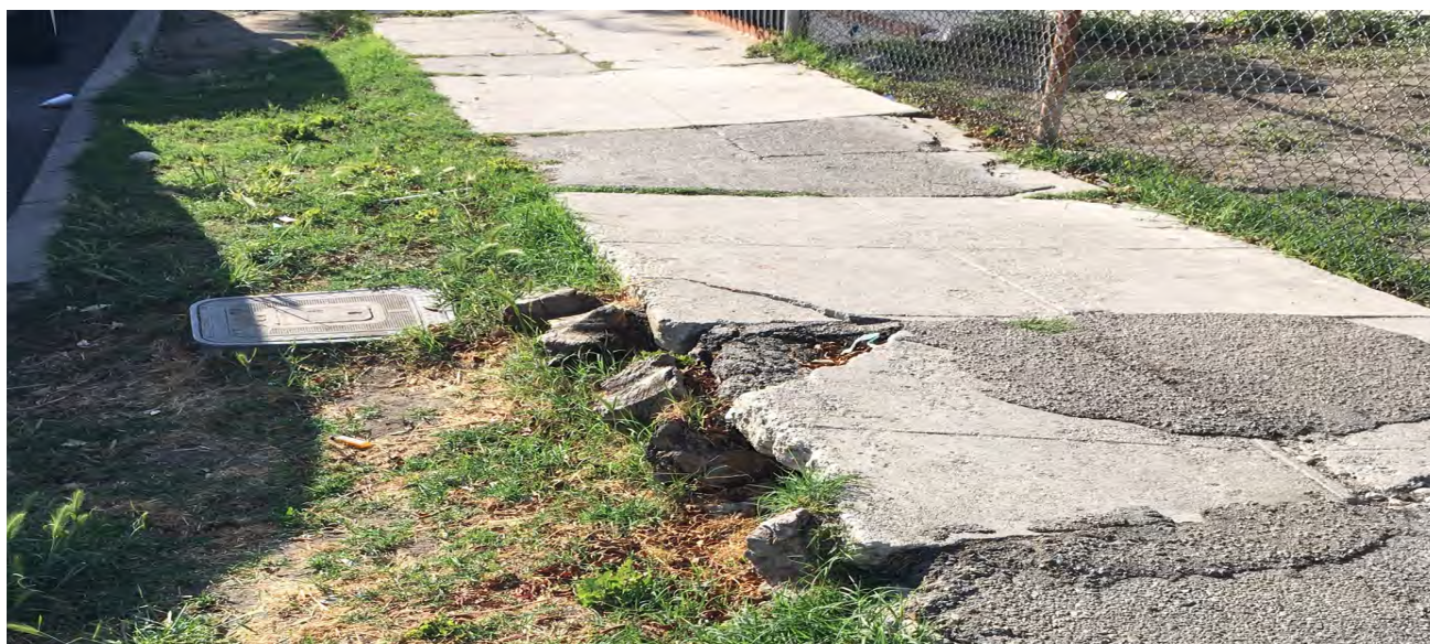
Top left: Underground utility box with large hole along Central Avenue. Top right: Narrow sidewalks on East Adams Boulevard do not provide enough space for a pedestrian using an assisted mobility device and often force pedestrians into the sidewalk buffer and the street. Bottom: Uneven and uplifted narrow sidewalk along East Adams Boulevard create a tripping hazard.
