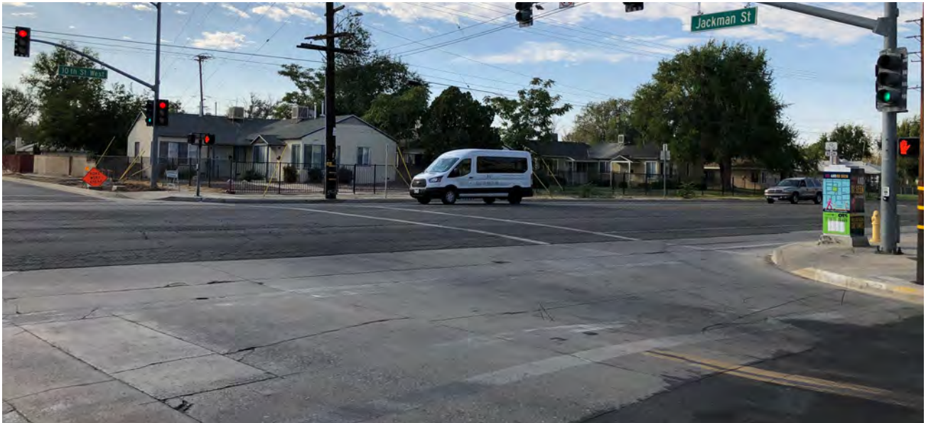
Faded crosswalk markings on West Jackman Street and 10th Street West.
