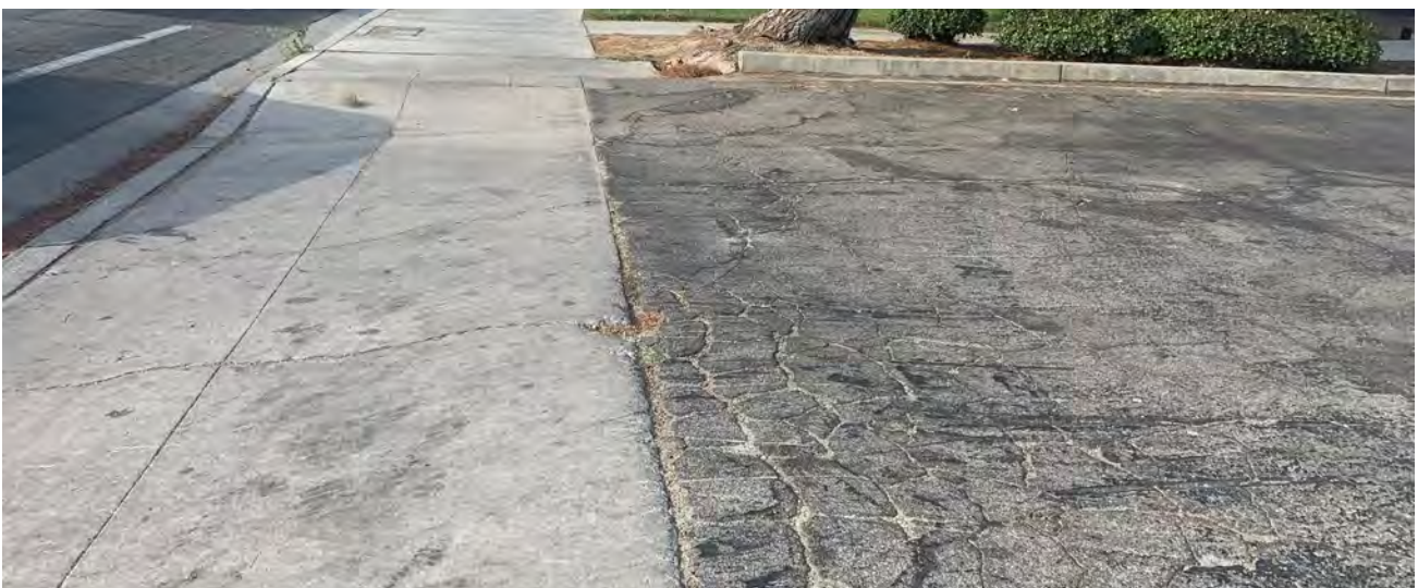
Top: Cracked roadway and lack of sidewalks on 10th Street West, between West Jackman Street and West Lancaster Boulevard. Bottom: Poor pavement condition at the entrance to businesses on 10th Street West.
