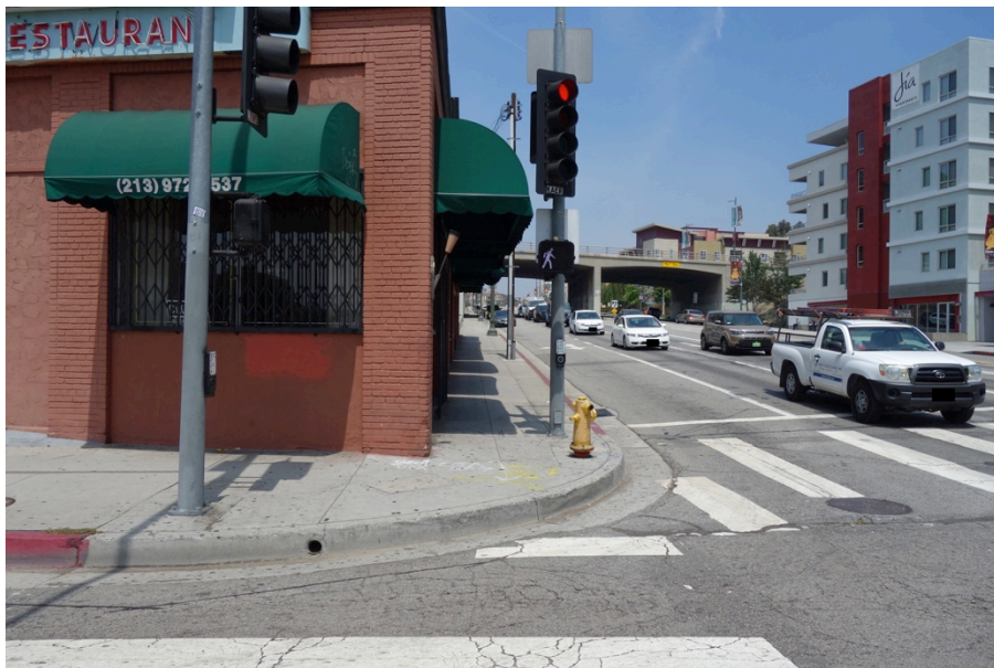
HIGH CURB AND LACK OF CURB RAMP AT N. BROADWAY AND CESAR CHAVEZ AVENUE
