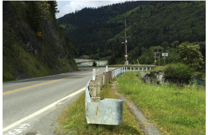
CLEARLY WORN PEDESTRIAN PATHS ALONG THE SIDE OF SR-96 IN THE BLUE SLIDE SECTION; ERODING SECTIONS OF THE INFORMAL PATH EXPOSE PEDESTRIANS TO DANGEROUS CONDITIONS
