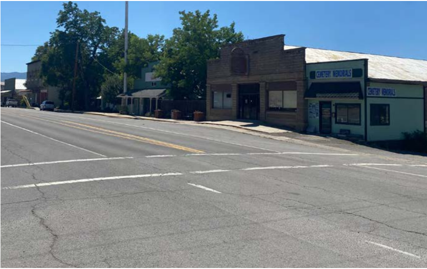
Faded crosswalk markings on Main Street (SR-3) at Sterling Street
