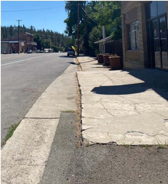
Cracked and uneven sidewalk in front of The Creamery
