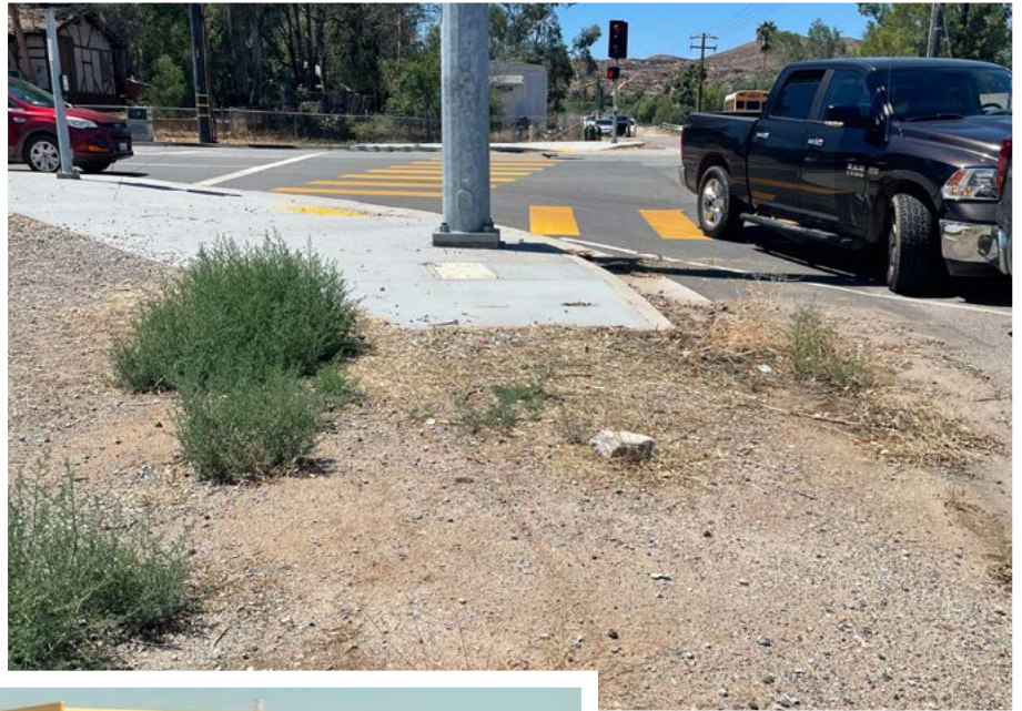
RIGHT: Incomplete sidewalks on the southeast corner of the Garbani Road/Murrieta Road intersection.
