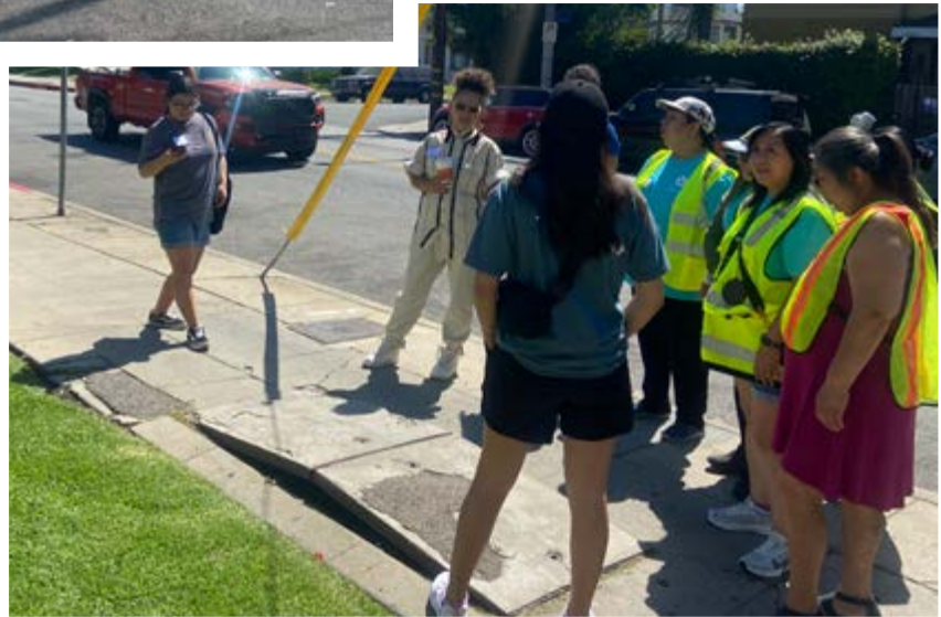
ABOVE: Community members stand near a ramp that has been erroneously created on the sidewalk.
