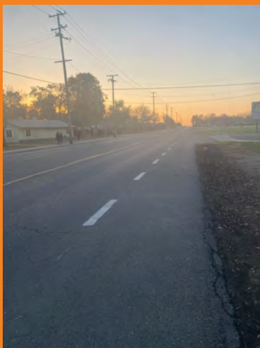
IMAGE: EXISTING BIKE LANE AT THE NORTHSIDE OF EAST CALIFORNIA AVENUE, BETWEEN WATERMAN AVENUE AND KERN STREET
