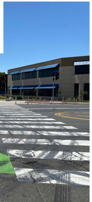
TOP: The Ohlone Greenway connects to Central Avenue, providing a north to south multi-use trail between Berkeley and Richmond. MIDDLE: Carlson Boulevard/San Pablo Avenue crosswalk which features hazards like uneven bricks and construction plates. BOTTOM: Rydin Road/Central Avenue intersection, full of tire marks from dangerous driver behavior.
