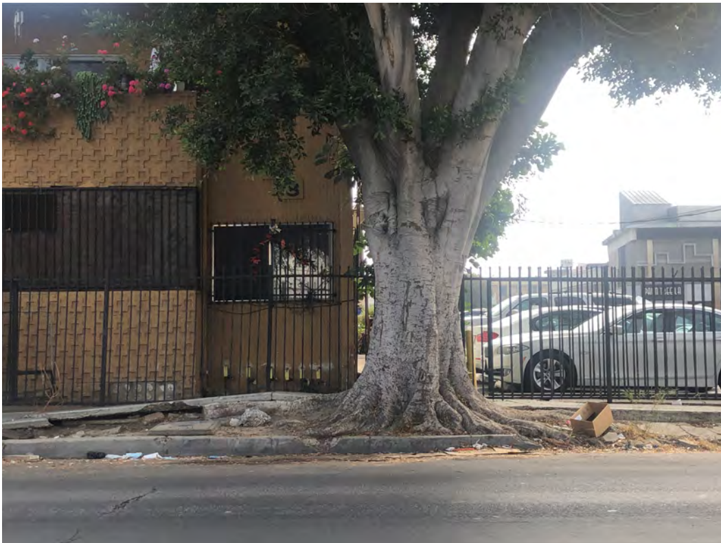
An uprooted sidewalk from a large tree near Hobart Elementary School.
