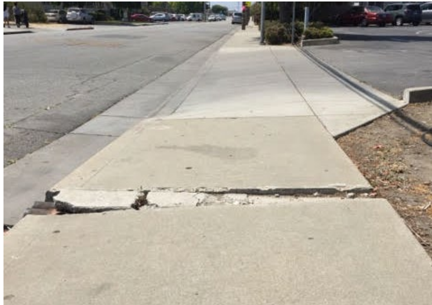
Large crack in sidewalk on Alta Vista Avenue was a reported barrier for community residents who rely on an assisted mobility device.
