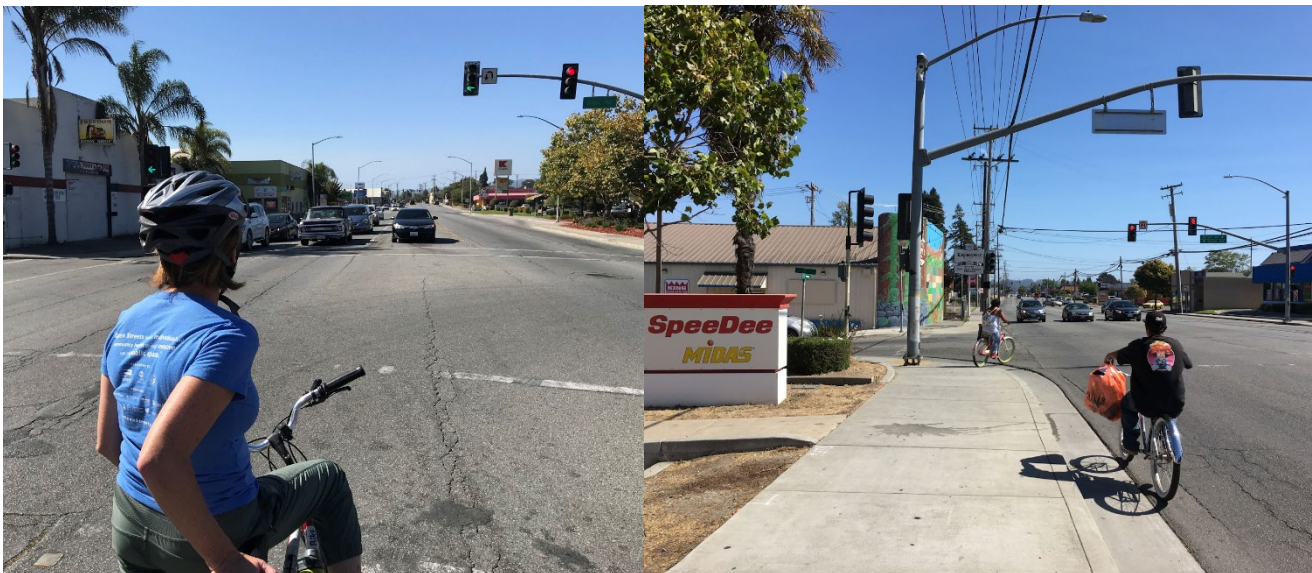
Road maintenance and repair needs as visible from a bicyclist perspective traveling north on Freedom Boulevard and Davis Avenue Intersection (left). The lack of bicycle facilities along Freedom Boulevard creates opportunities for unpredictable and potentially unsafe bicyclist behaviors (right).
