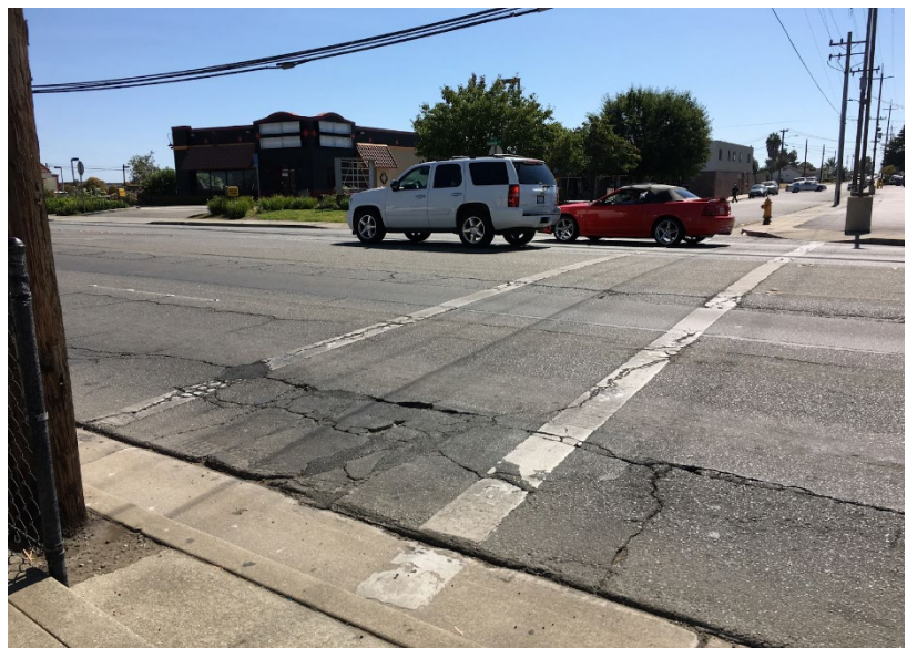
At Freedom Boulevard and Mariposa Avenue: No pedestrian crossing signage is present, there is no curb ramp on the east side of the crossing, and utility poles block part of the crossing and visibility of oncoming motorists.
