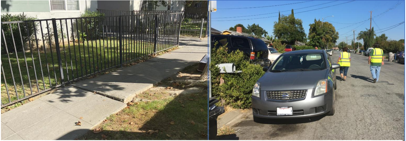
Root heaves like this are common on the narrow sidewalks on Appian Lane. Sidewalks are detached and separated by landscaping (left). In the Bonita neighborhood, the sidewalk network is disconnected, with many missing segments, including on Lotus Street and Herald Avenue (right).
