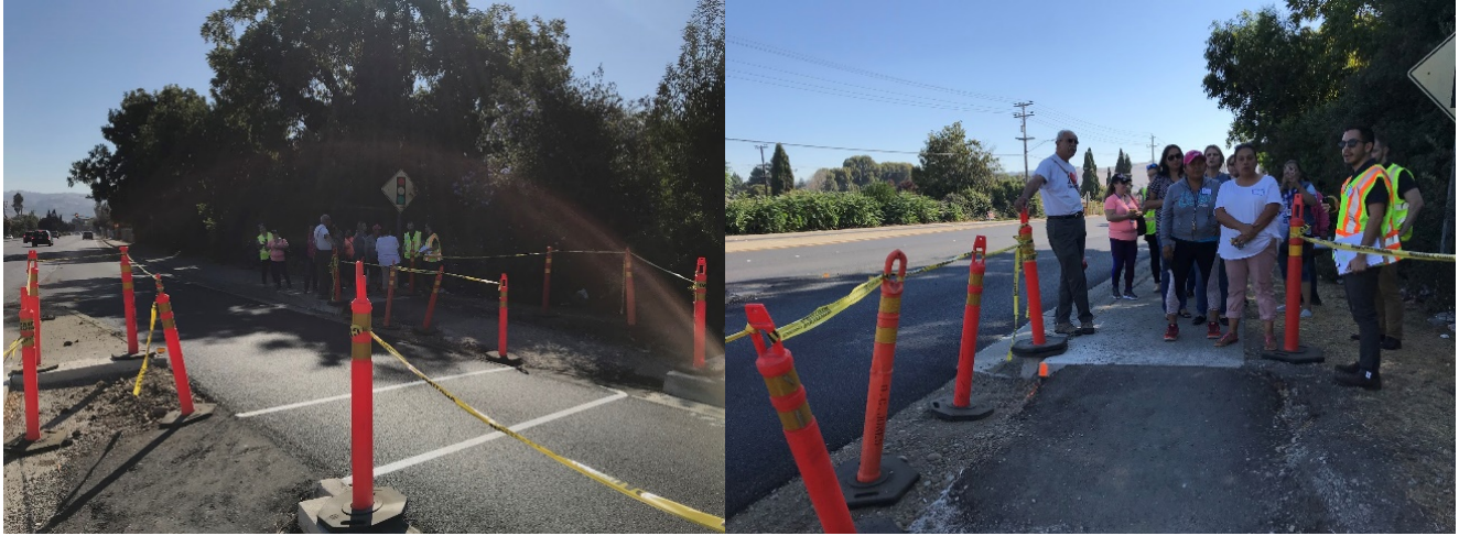
Construction zones at Tennyson Road and I-880 create barriers for pedestrians and community members who require mobility assistance devices.
