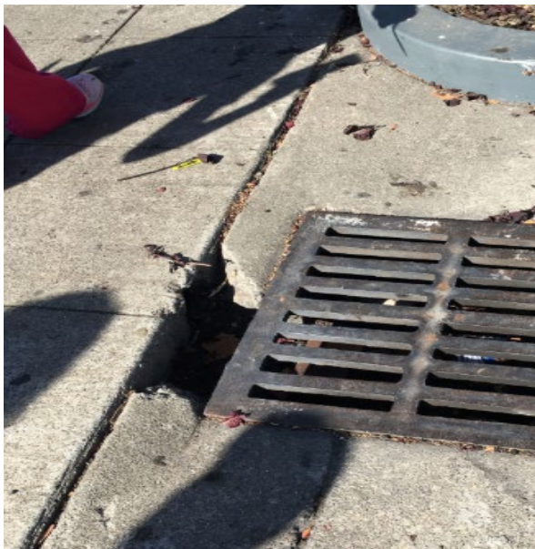
Large hole along the gutter and drain on westbound Tennyson Road. Participants observe how an older adult or someone using an assistive device or stroller can get stuck and hurt.
