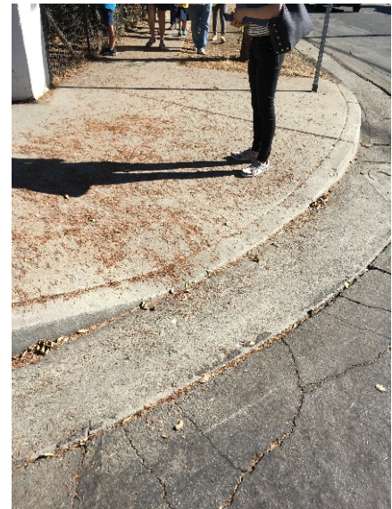
During the Site Visit and workshop participants noted a number of missing or older ADA ramps within the community.
