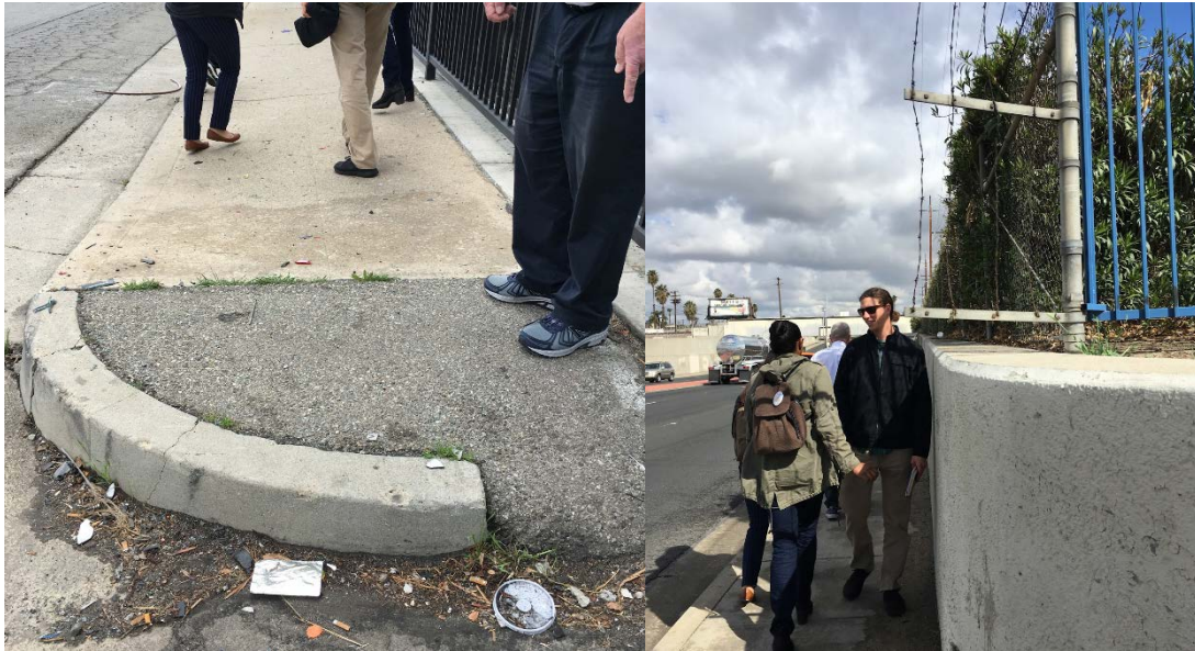
Sidewalk conditions along SR 204 are narrow and lack ADA ramps.
