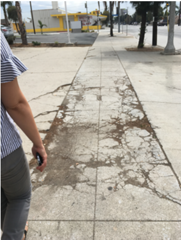
Extremely cracked sidewalk creates a hazard for pedestrians and bicyclists using the sidewalk.
