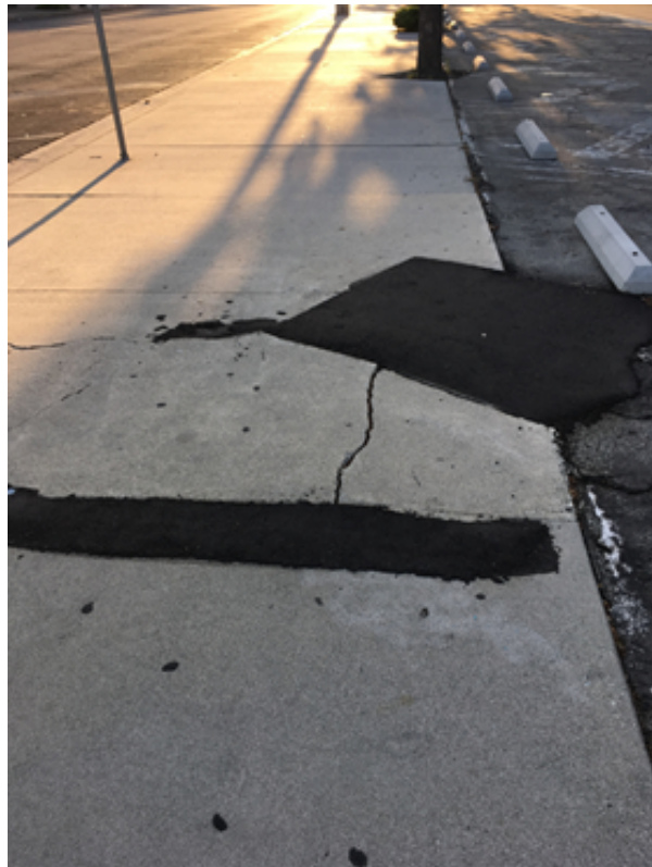
An upheaved sidewalk that has been repaired in patchwork fashion.
