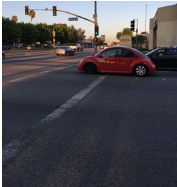
Faded crosswalk markings make it difficult for drivers to see and respect the crosswalk.
