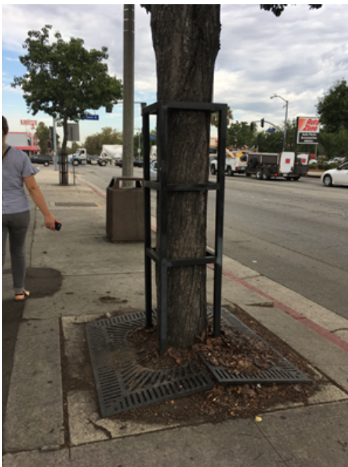
Tree wells filled with debris and uplifted from expanding tree routes.
