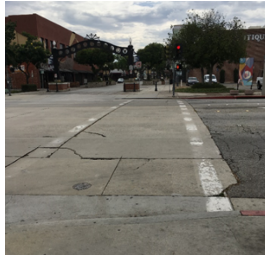
East Holt Avenue looking east towards North Gibbs Street is a wide multi-lane street with faded markings, cracked pavement, and potholes.
