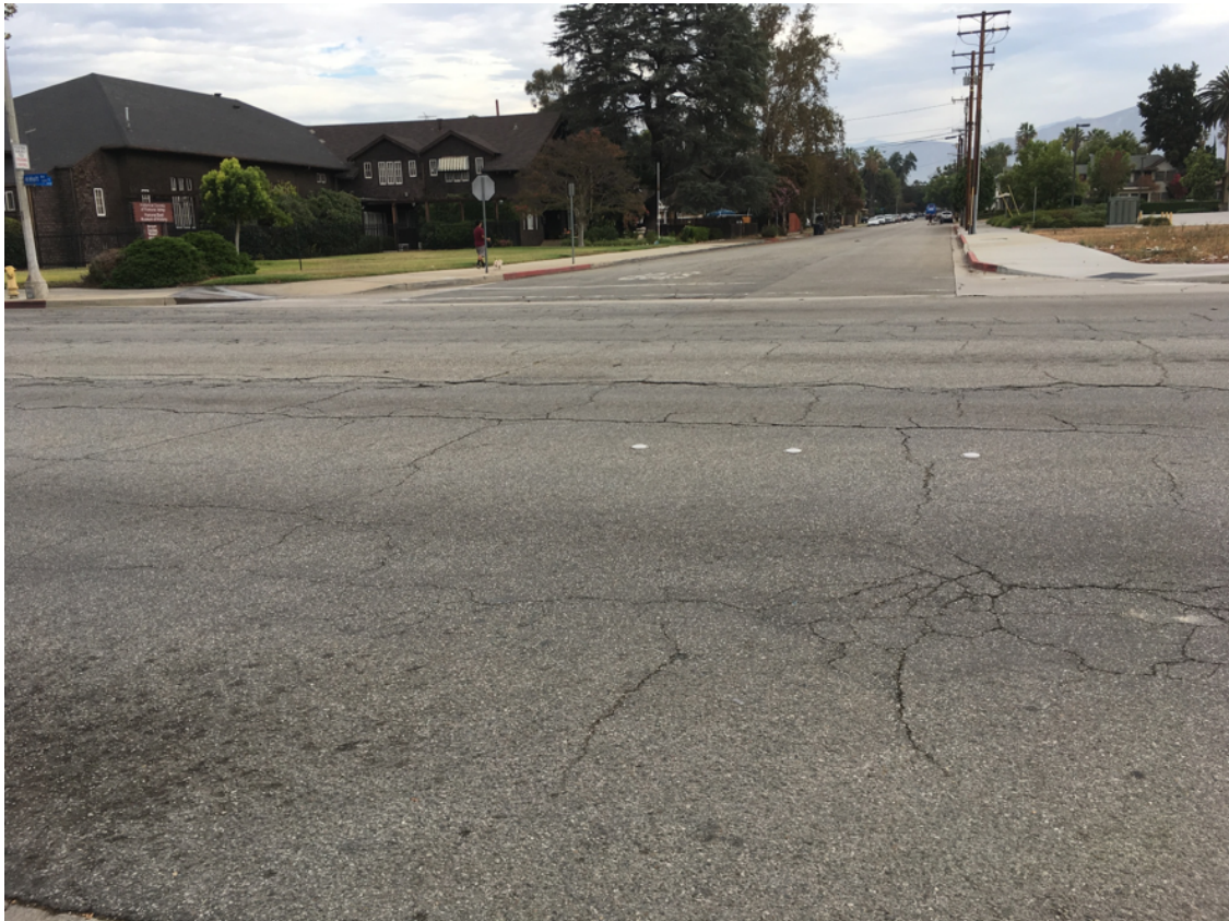
East Holt Avenue looking east towards North Gibbs Street is a wide multi-lane road that encourage speeding.
