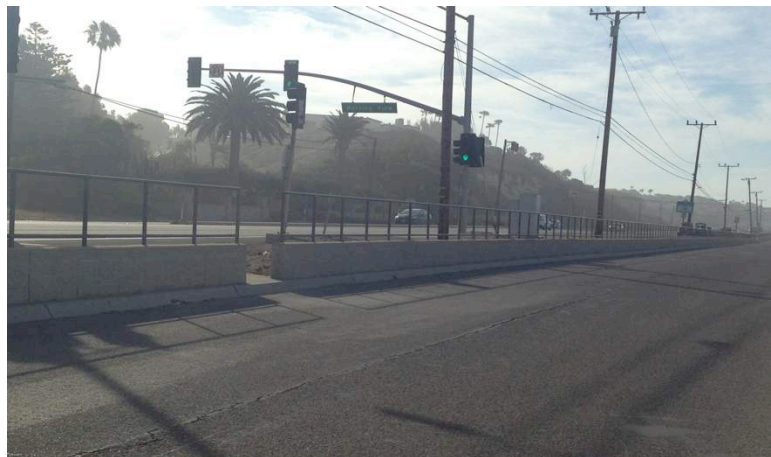
Figure 20: Pedestrian access point to Zuma Beach from Morning View Drive bus stop and crosswalk. The entrance is not wide and provides a step, rather than a ramp. (Caro Jauregui)
