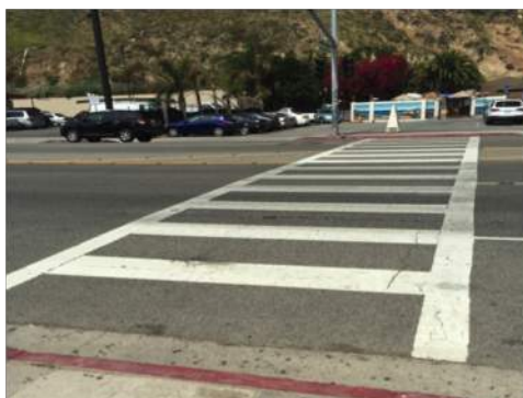
Figure 13: Lack of curb ramps at Malibu Pier crossing (Tony Dang)
